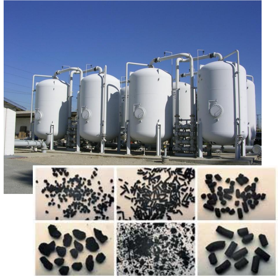
Potable Water Treatment
