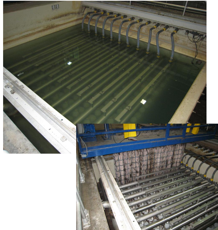
LOTT Martin Way Reclamation Plant MBR
